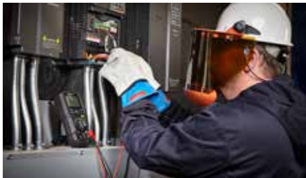
Troubleshoot Variable Frequency Drives using VFD mode
